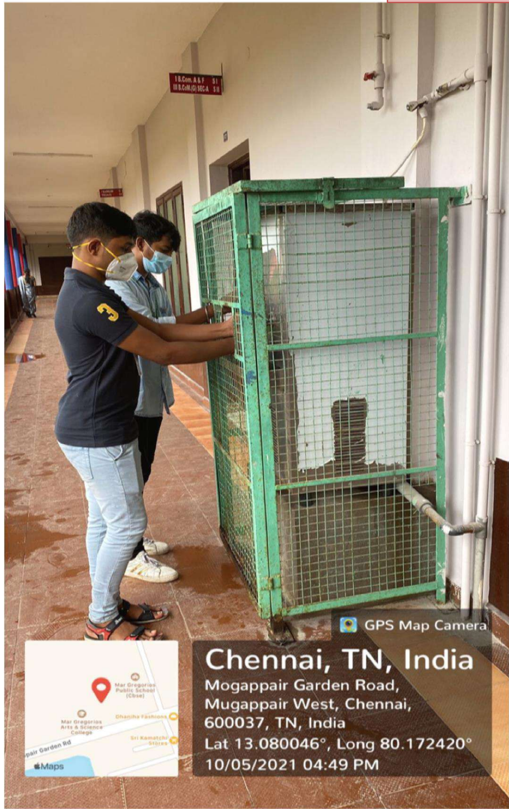
RO Drinking Water
